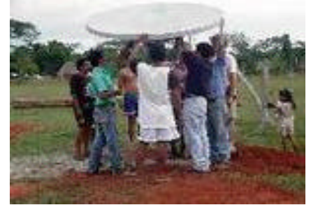
2000, PORVENIR, BOLIVIA: SolarQuest® and local students install the remote telecenter in collaboration with the White House Millennium Council using ICTs and solar energy.
