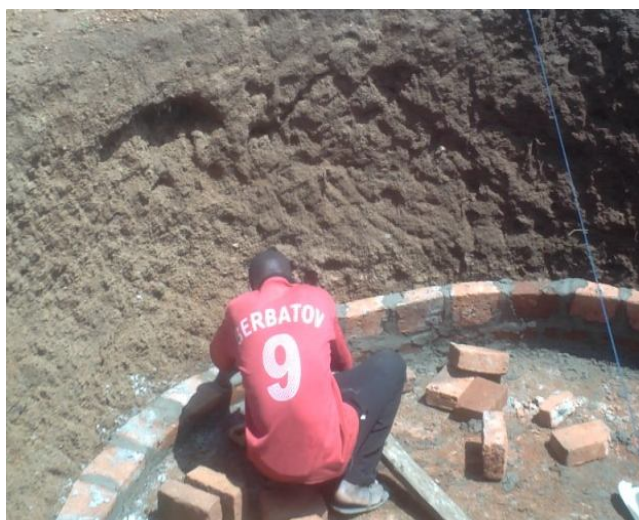
One of our biogas Masons installing a biogas digester in Kigingi, Nkondo – Buyende (2011)
