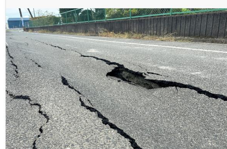
Road that has caved in / Kumamoto Prefecture / July 30, 2026 ©JPF
