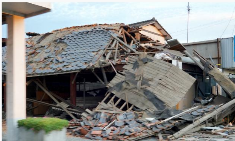
Houses destroyed by the earthquake / Kumamoto
