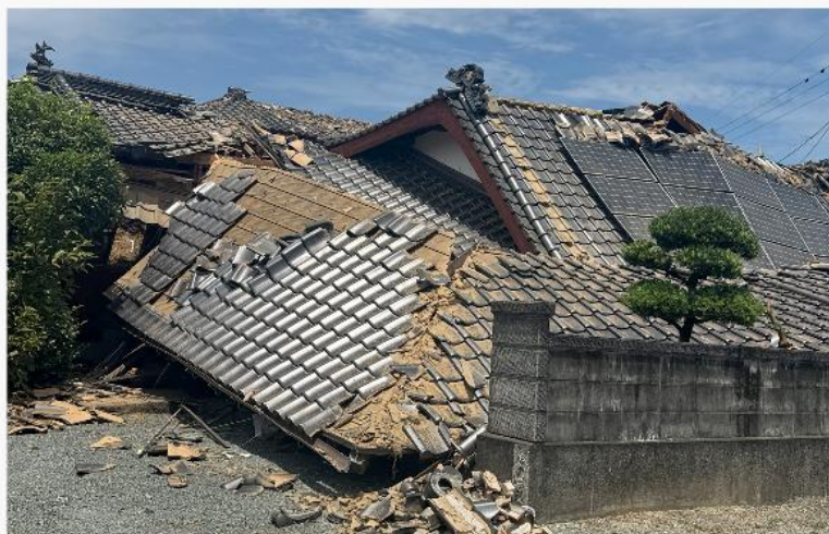
View of a house that collapsed due to the earthquake Kumamoto Prefecture / July 30, 2026 ©JPF
