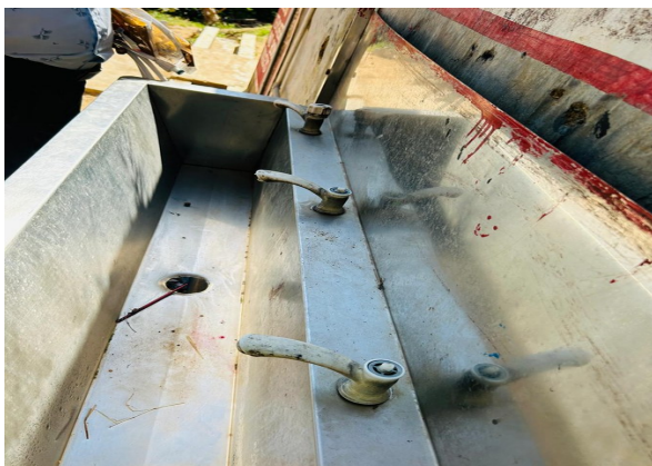
5. Existing school handwashing facility and old taps
