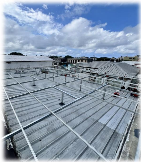
Stainless steel support structure.
