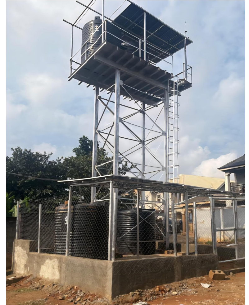
Eginrin Ekun Community Solar Powered Water Supply System
