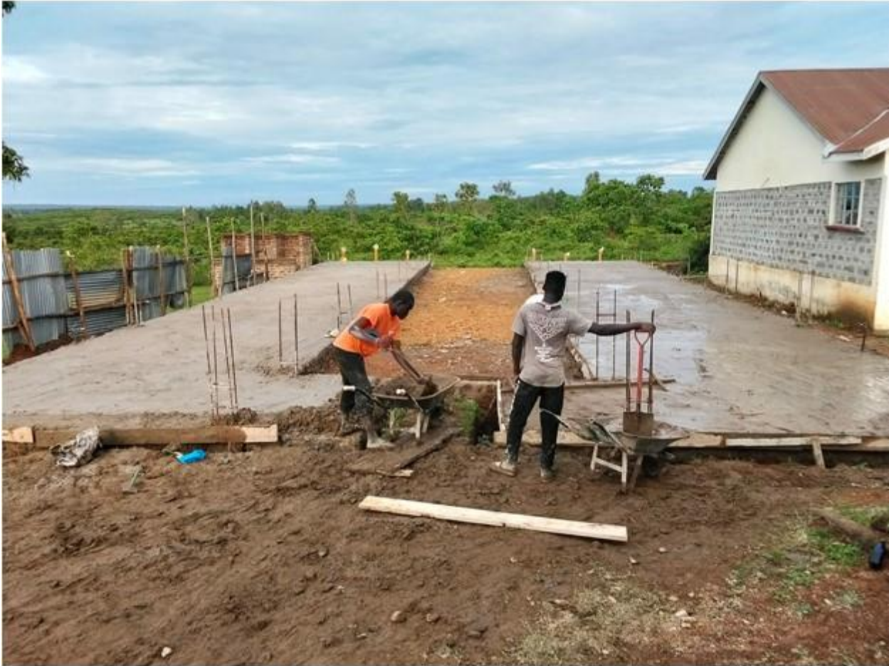
Boys' dormitory ground floor slab is near completion at the IoT main campus.
