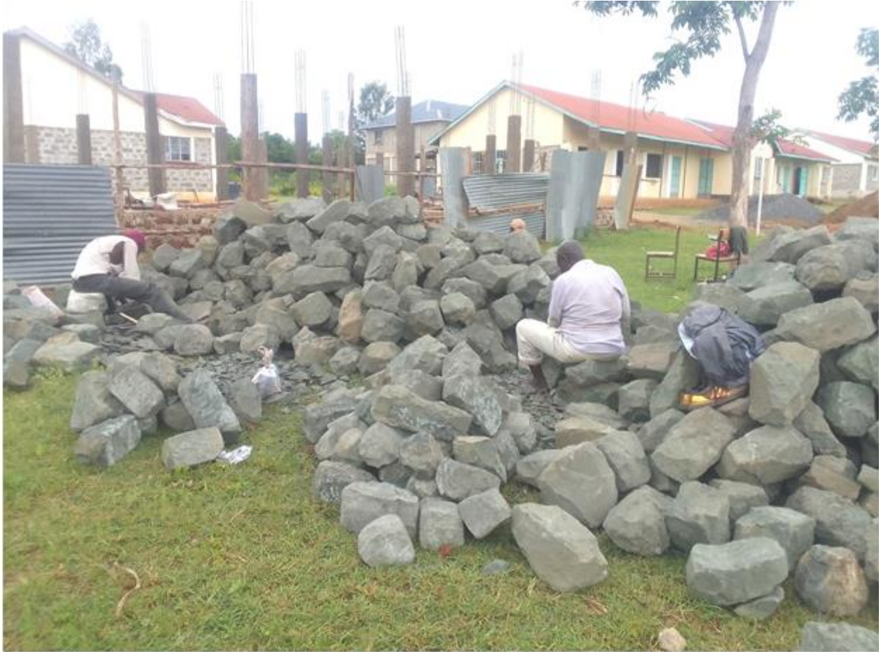
Stone dressing for the Boy's dormitory walling work is in progress at the IoT main campus.
