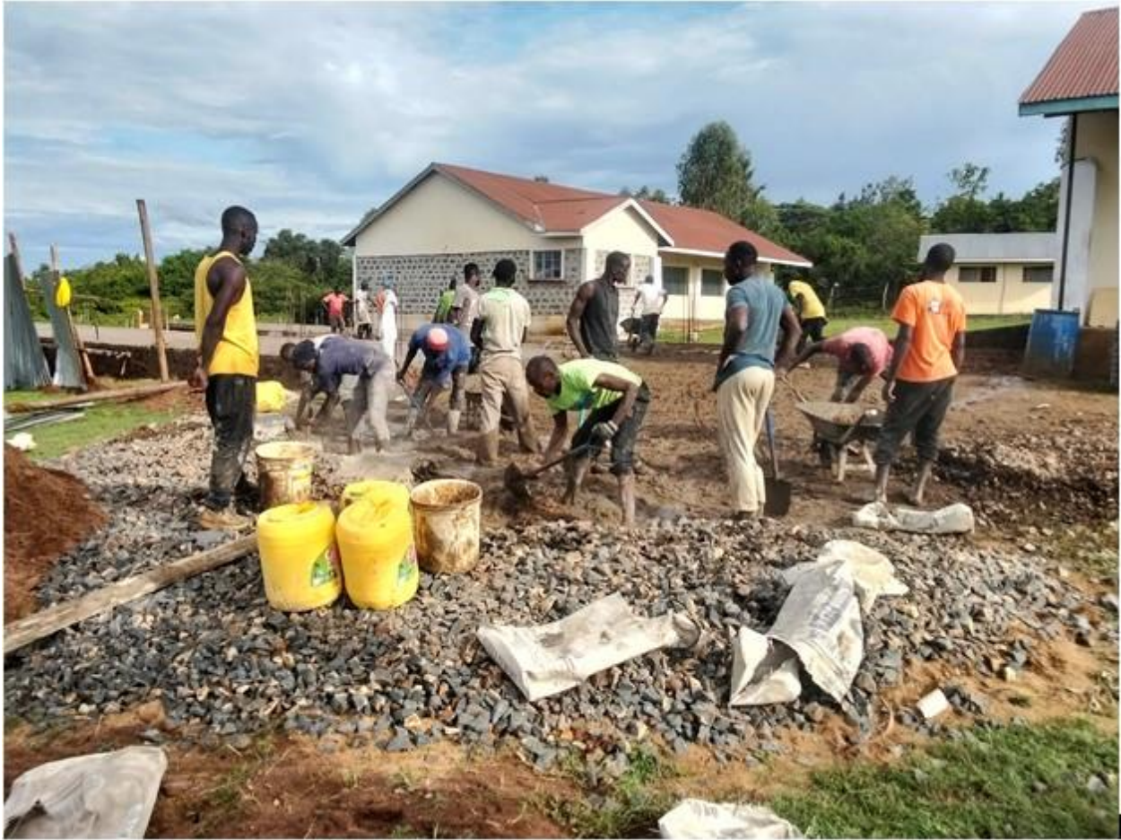
Boys' dormitory ground floor slab work is in progress at the IoT main campus.
