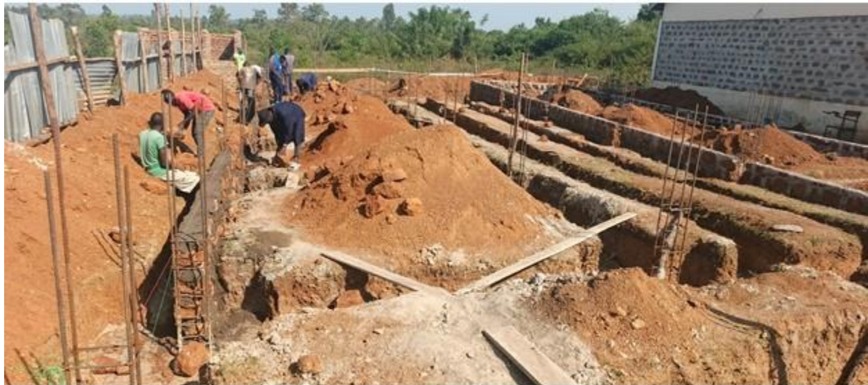
IoT Boy's dormitory wall foundation work is in progress at its main campus.
