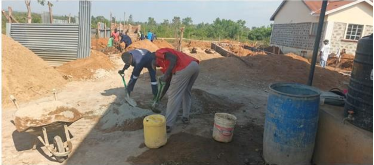
Building department students engagement in the construction work of boys' dormitory at the IoT main campus.
