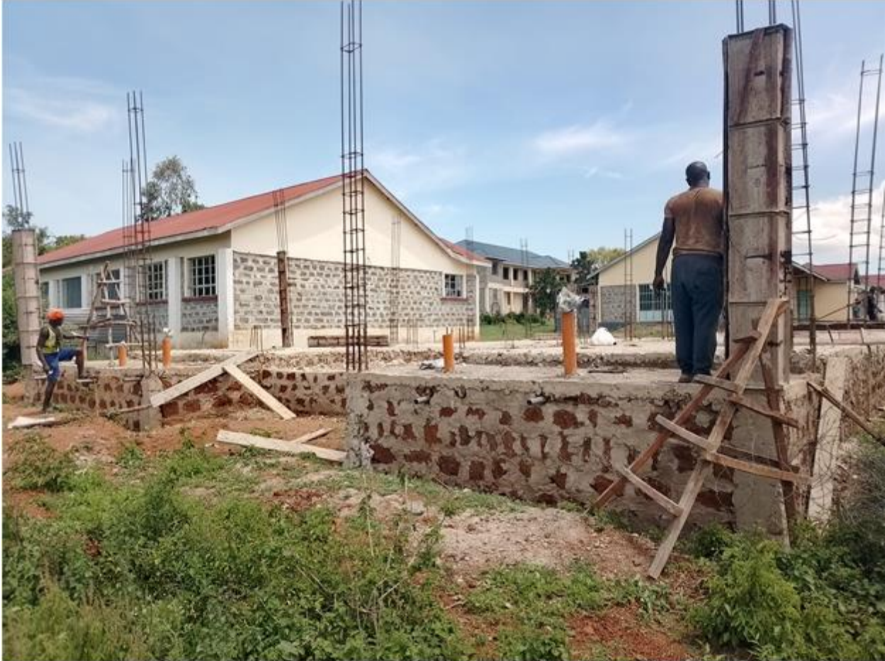
Erecting column bases for the Boy's dormitory at the IoT main campus.
