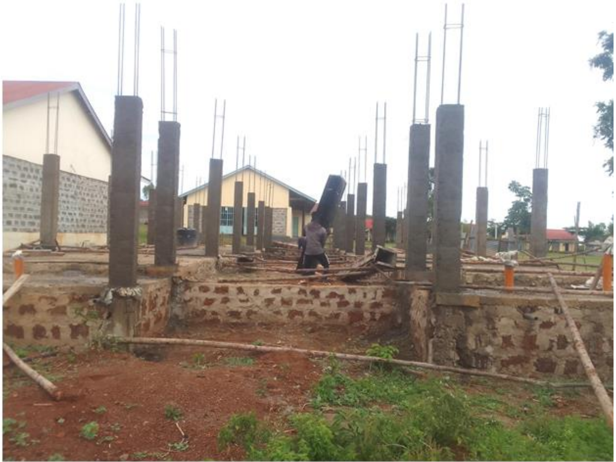
Column bases work is complete for the Boy's dormitory at the IoT main campus.
