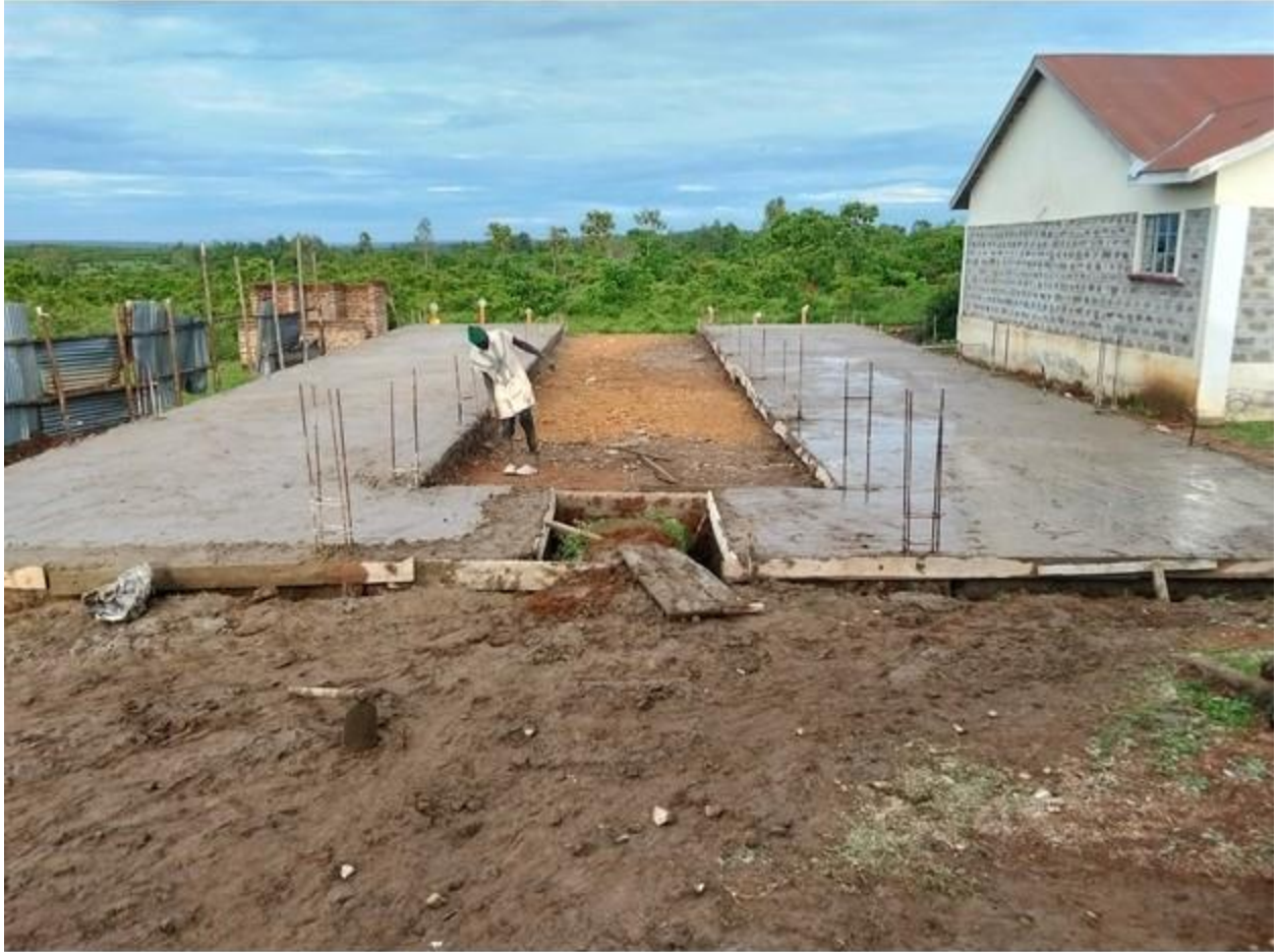
Boys' dormitory ground floor slab work is complete at the IoT main campus.
