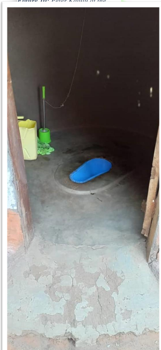
Figure 12: Sato pan inserted in the pit latrine
