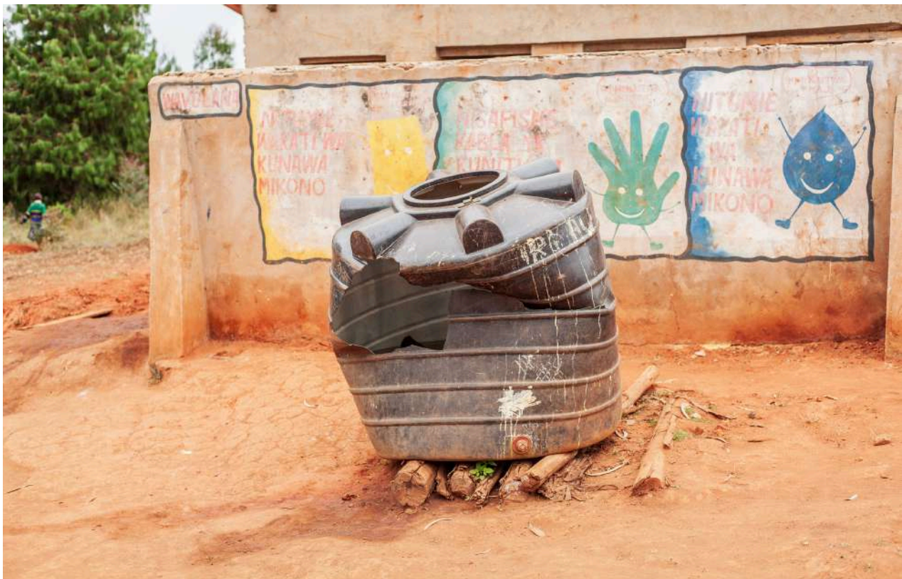
Toilet water storage facility at Luhindo Primary School is in a critical state, highlighting the urgent need for intervention.
