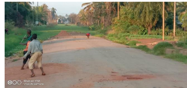
A number of infrastructures have been damaged and cause the community members face challenges on transportation, leading to increase of living costs
