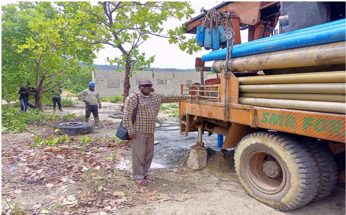
Drilling of wells on the site of the new Koumoniadè health center on April 8, 2024
