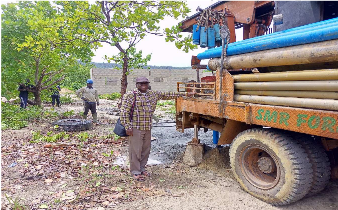
Drilling of wells on the site of the new Koumoniadè health center on April 8, 2024
