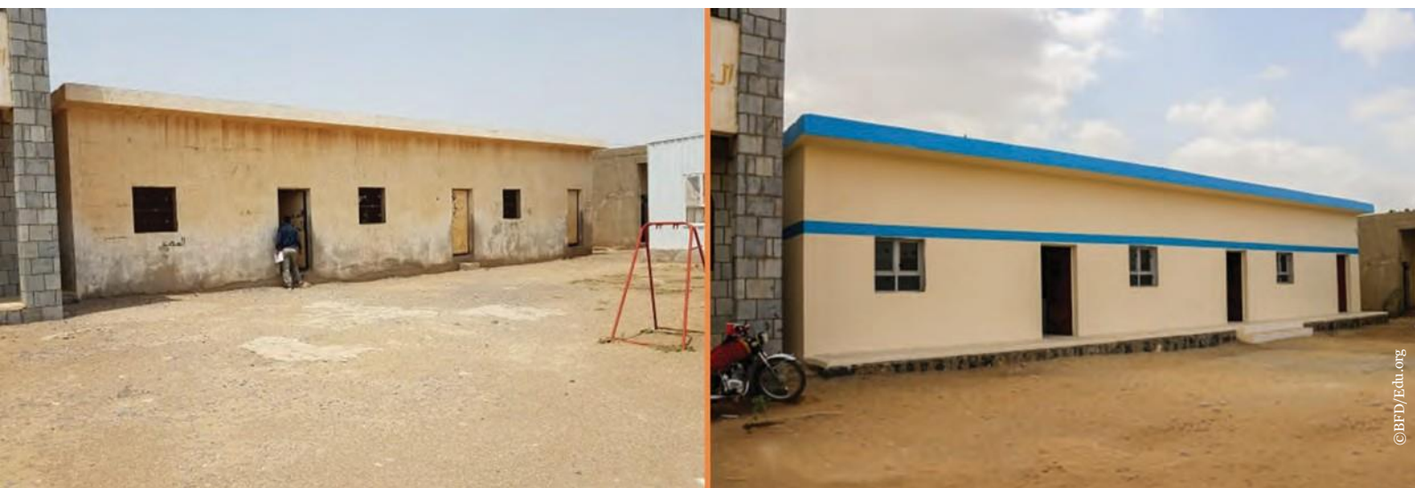
Location: Om Salamah School – Before and After the Intervention – Al Qanawis District – Al Hudaydah Gov.
