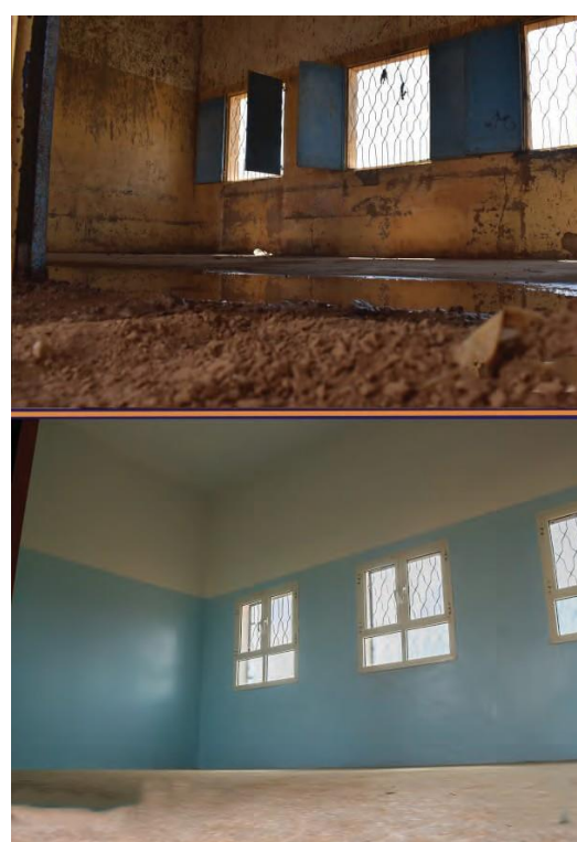
Location: Al-Noor School – Before and After the Intervention – Al Qanawis District – Al Hudaydah Gov.
