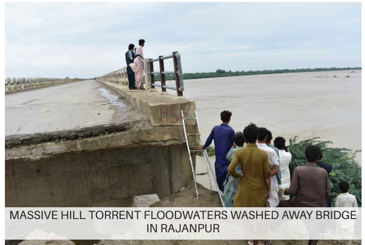
FLASH FLOODS DISCONNECTED ROAD LINK BETWEEN KARACHI AND QUETTA, BALOCHISTAN
