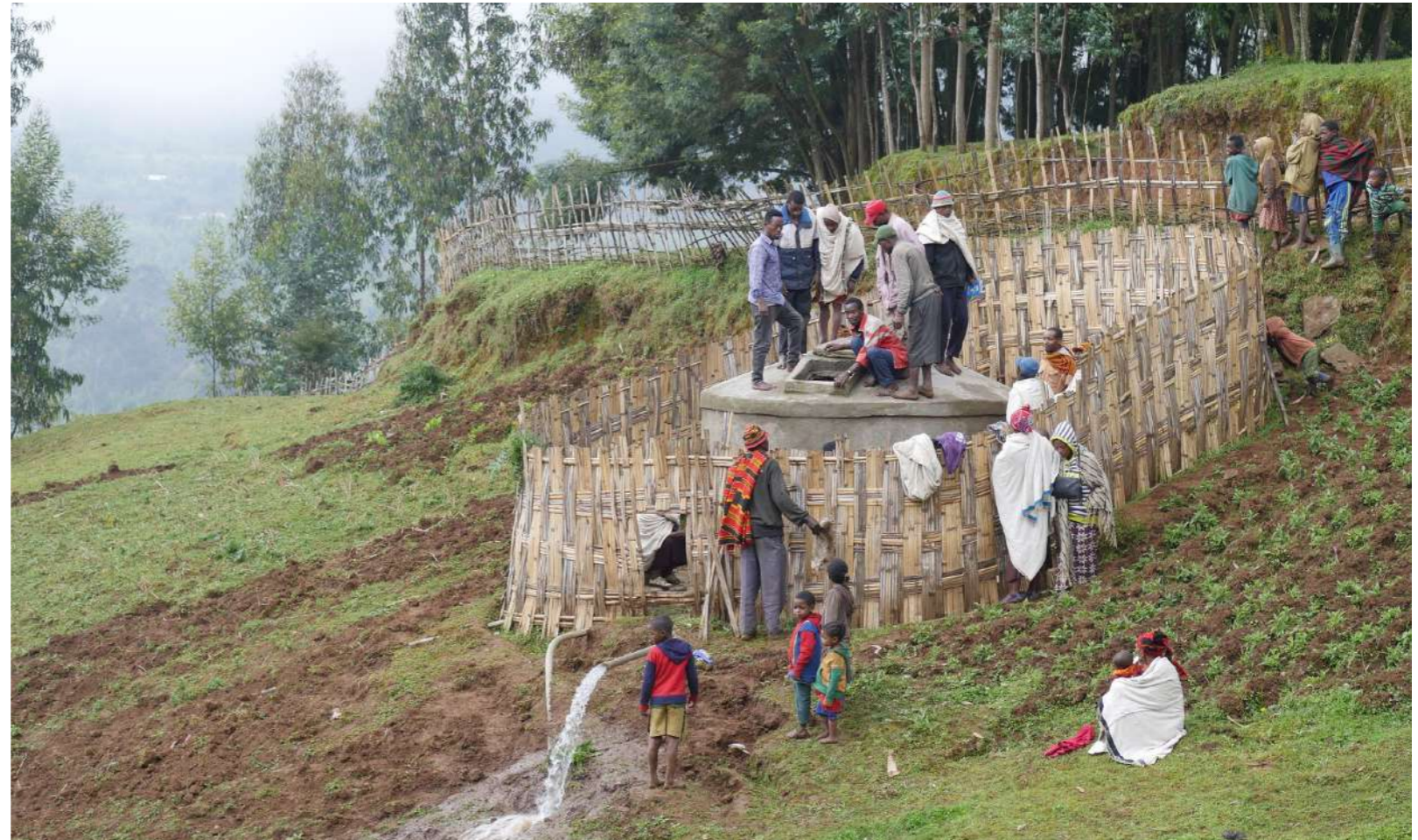
The maintenance team and the committee members training on water reservoir maintenance
