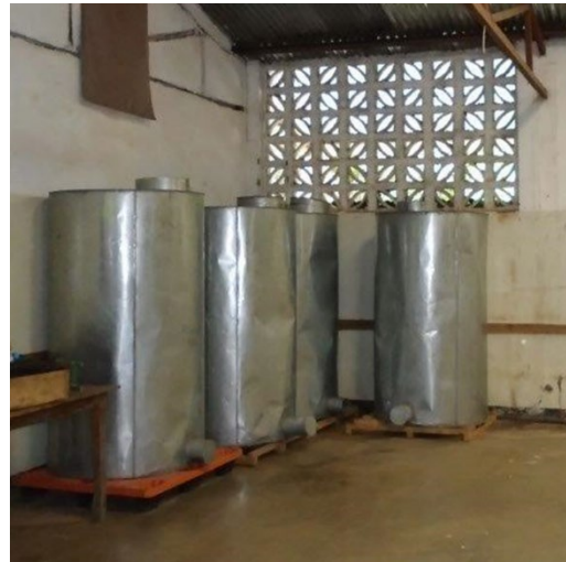
Photo 3 Silos for effective storage
