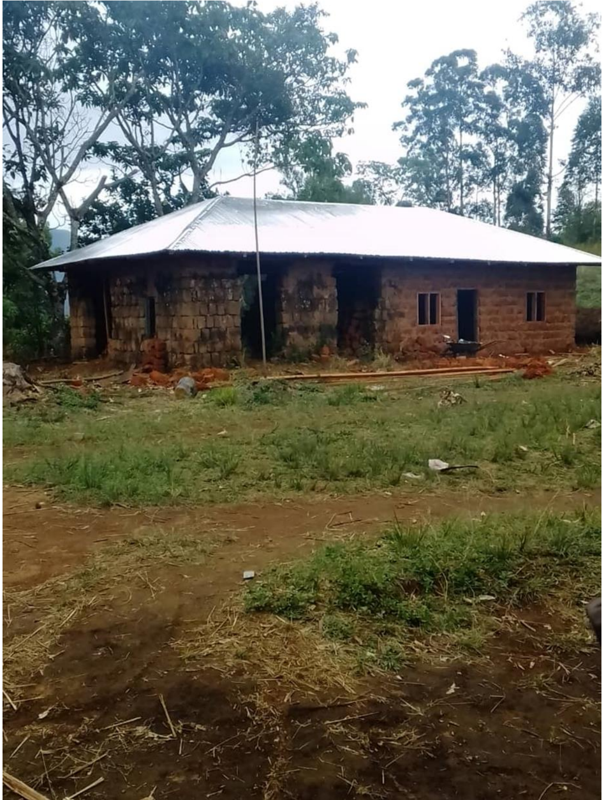
RECEADIT New Building under Construction for the lodging of the Internally Displaced People, RECEADIT Medical workers, Clinic Canteen and Food Store for both the Ngemsibo Community members and our Clinic Medical Workers
