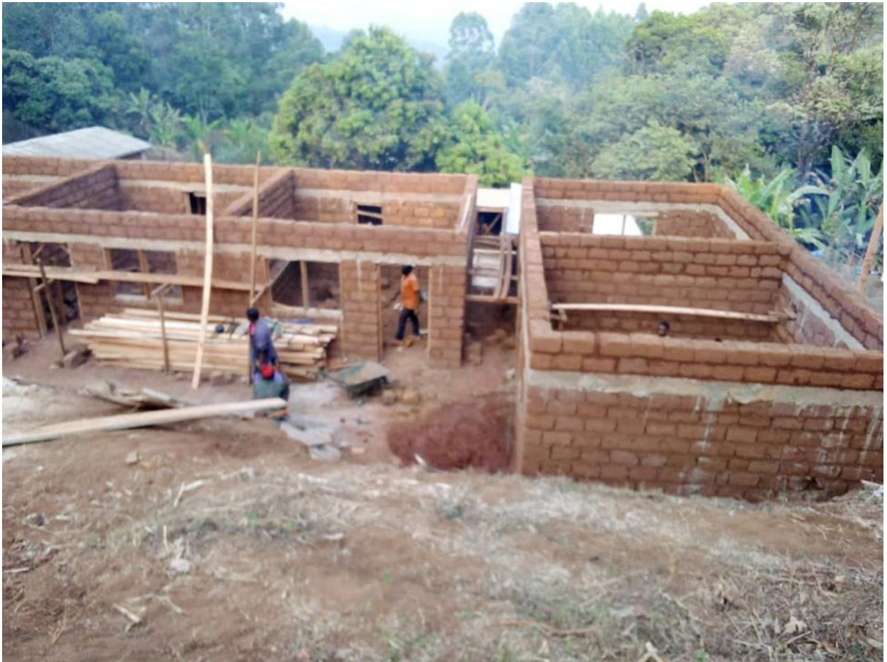
RECEADIT New Building under Construction for the lodging of the Internally Displaced People, RECEADIT Medical Workers, Clinic Canteen and Food Store for both the Mbam Community members and our Clinic Medical Workers
