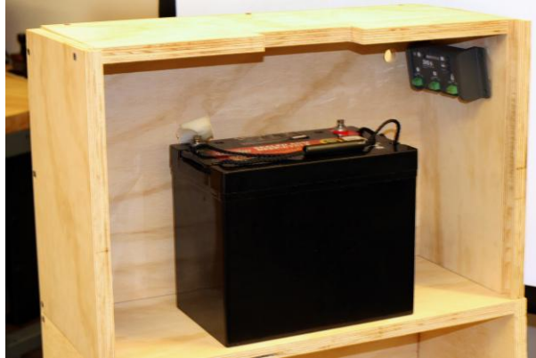
Figure 10: Battery and charge controller inside battery box
