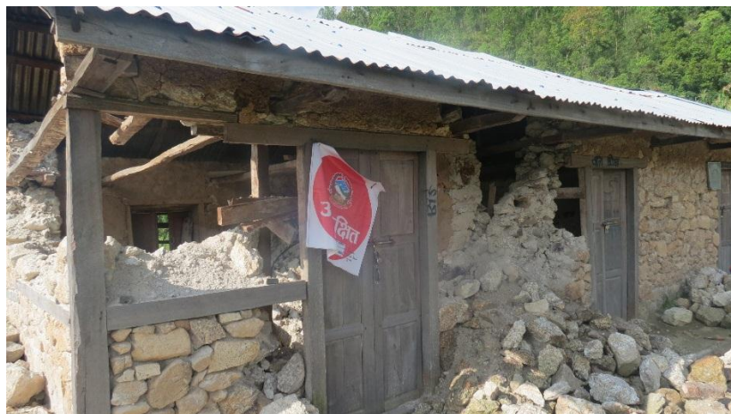
Figure 1 A damaged building of Rastriya Primary School Alchhe, Dadakharka
