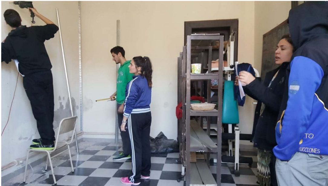
One of the buildings that needed repair, and the group at work.
