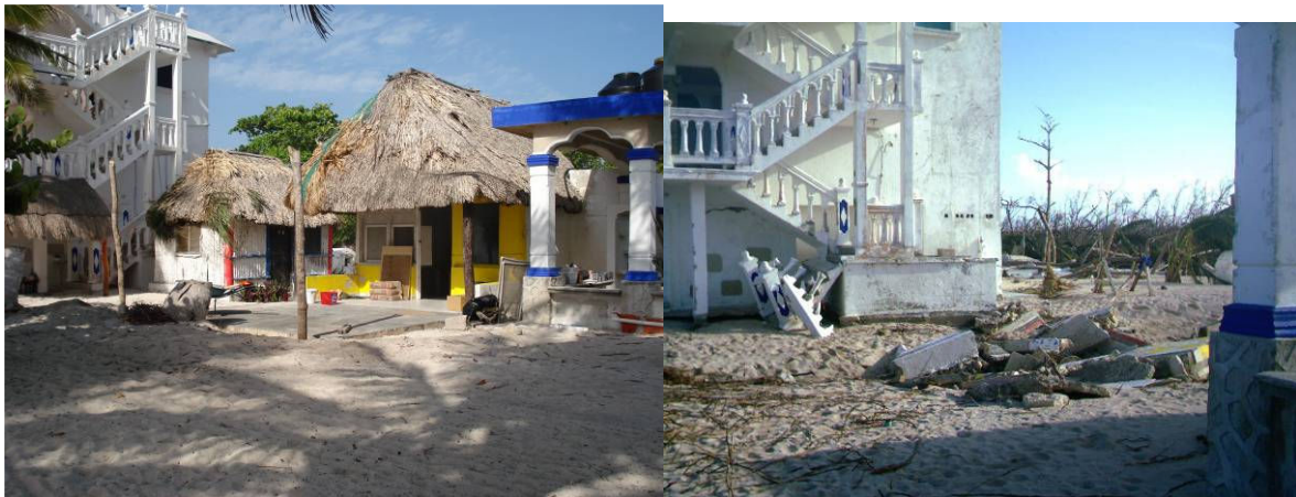
Destruction even of concrete structures.
