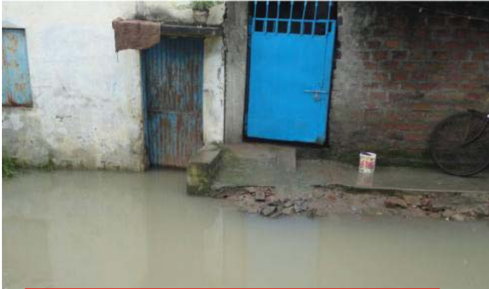
Rain water enters house
