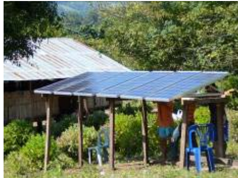
Solar Panels at DPN Hospital
