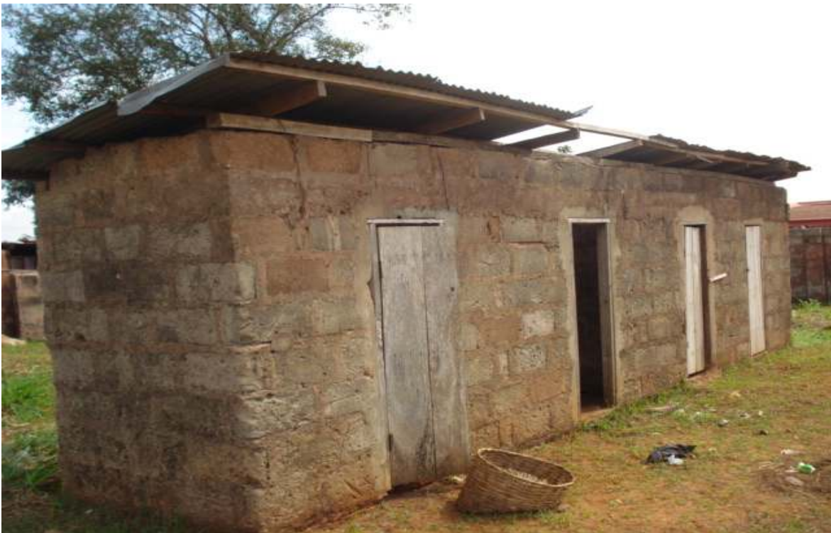
Dilapidated block of toilet building at community primary school Ugbolu
