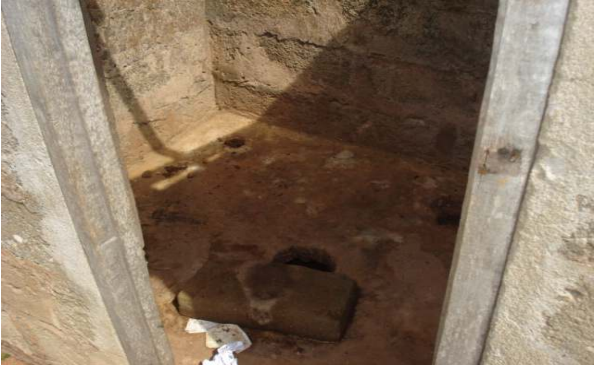
Interior of a typical ground toilet and the floor Condition of the toilet
