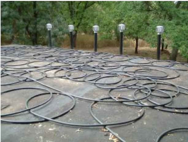
Solar heating coils March 2007
