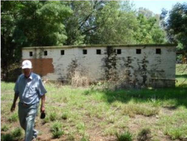
Derelict Ablution Facility before reconstruction Brian LaTrobe in foreground – Nov 2006
